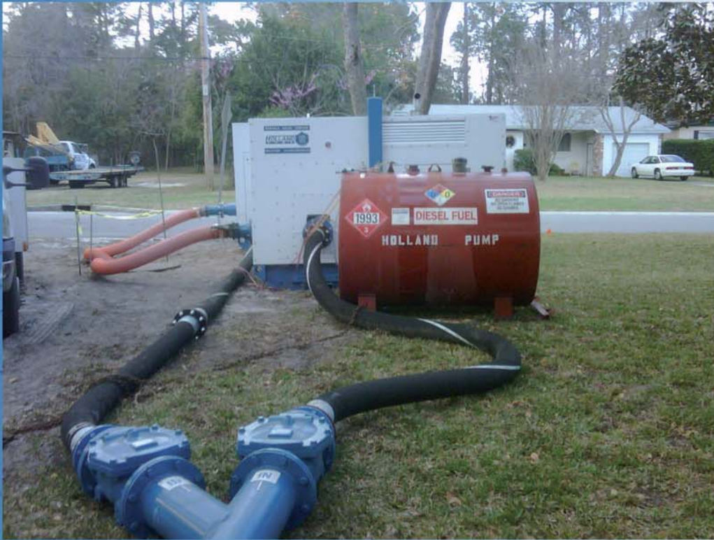
The Holland PT8TPC Super Silent Pump was approved by the neighbors on Conga Street.
